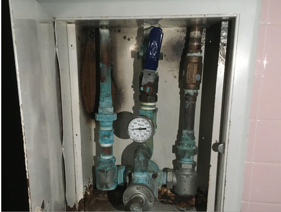
Deteriorating Galvanized Pipes
