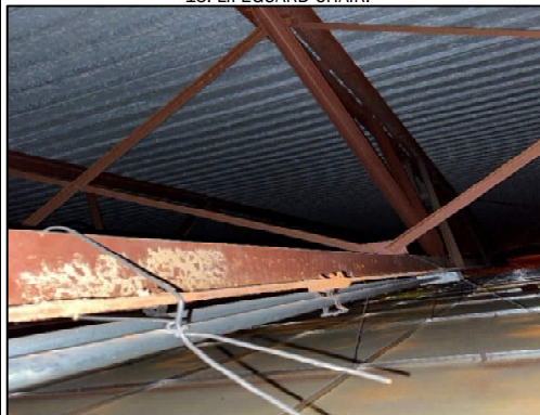
17. CORROSION ON DROP CEILING SUPPORT.
