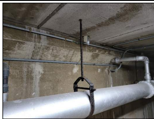
22. CORRODED PIPE HANGERS.
