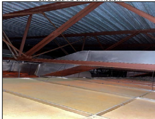
18. CORROSION ABOVE THE DROP CEILING.
