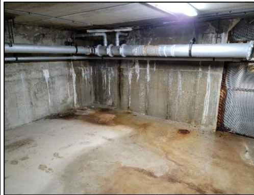
19. LEAK ON SOUTH SIDE OF DEEP WELL
