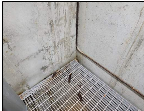
48. CORRODED CONDUIT SHEATHING ON THE FLOOR.
