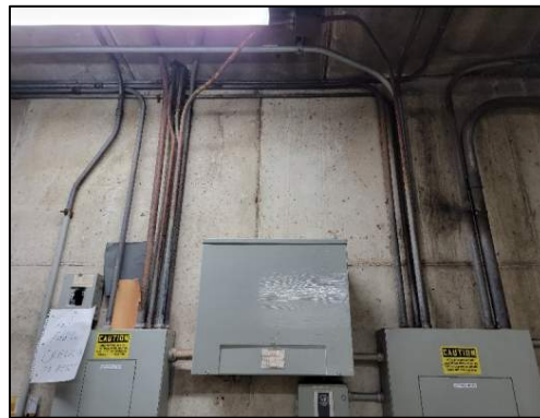
46. CORROSION ABOVE ELECTRICAL PANELS.
