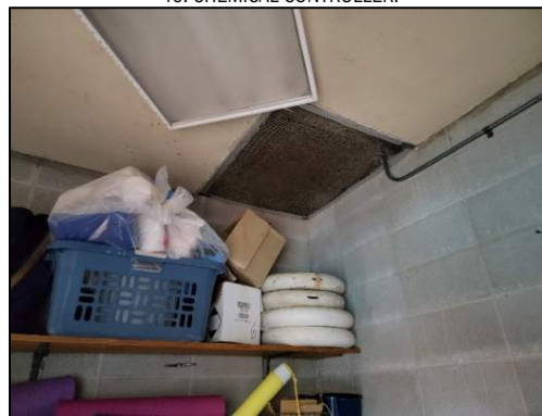
42. HVAC RETURN IN SUPPLY CLOSET.
