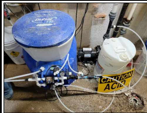
39. CHEMICAL FEED SYSTEM.
