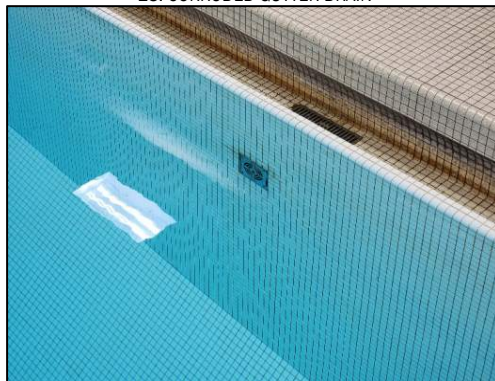
25. CORROSION AROUND AND ON INLET PLATE.
