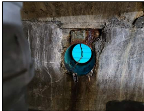
28. LEAKING AROUND LIGHT NICHE.
