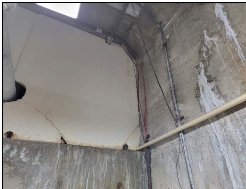
47. EXPOSED WIRES ABOVE SURGE TANK.
