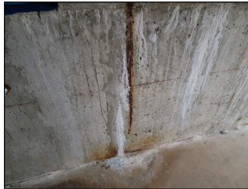
20. PRECIPITATE ON POOL BASIN WALL.
