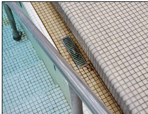
23. CORRODED GUTTER DRAIN
