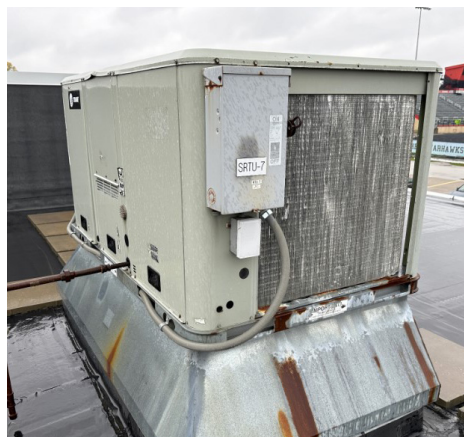
Failing HVAC System
