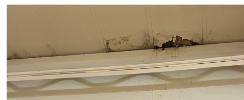
Deteriorating Gymnasium Ceiling
